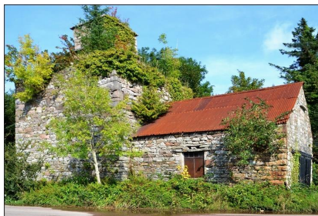
The furnace in the village of Furnace is now deteriorating, and its condition is of great concern to the villagers
