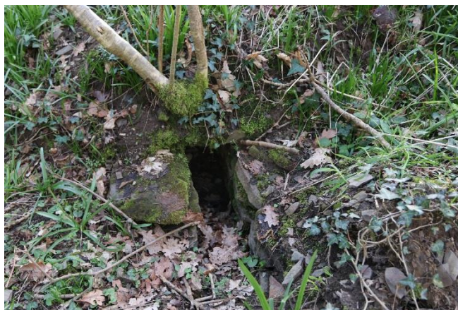
Plate 8 - The small stone "drain" on the western side of the brook – purpose unknown
