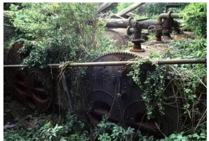
Two Lancashire boilers have deteriorated and the boiler house roof is very largely gone (Chris Allen / CC BY-SA 4.0)
