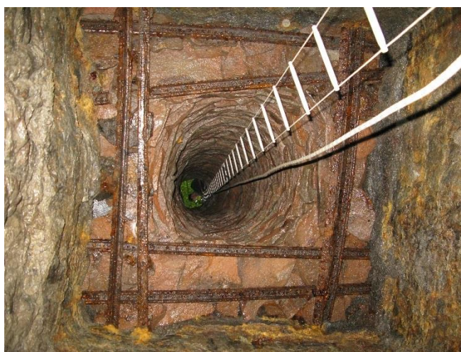
Plate 9 – Looking up the well from the bottom, the arrangement of the rails holding up the narrower round "ginging" are clear in this view
