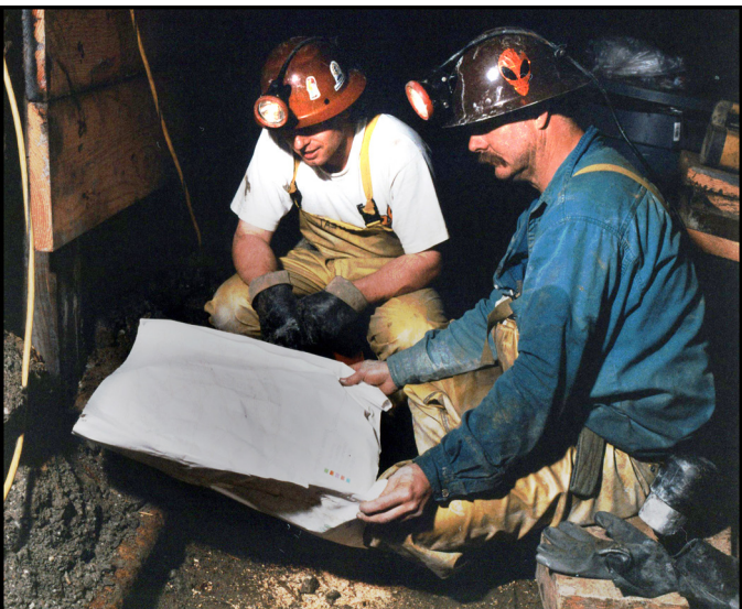
Fig 05 At the rock face, the supervisor and his colleague discuss the work to be done after lunch.
